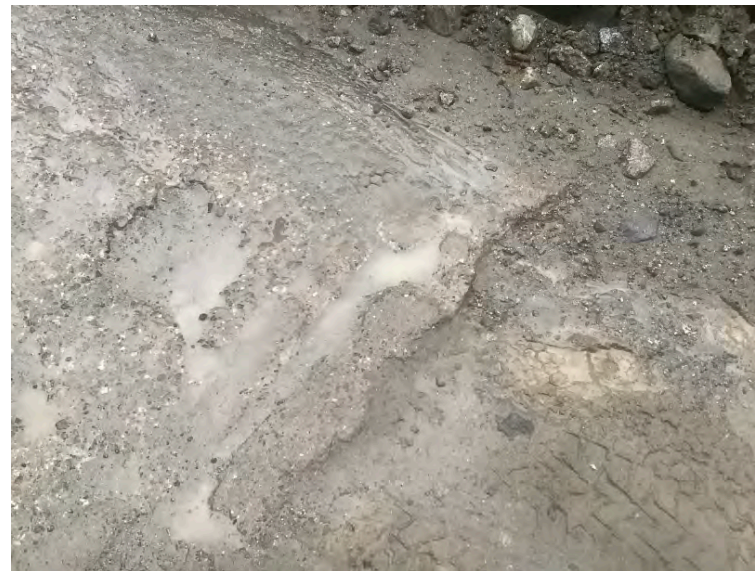
Downstream right top ballast wall damage
